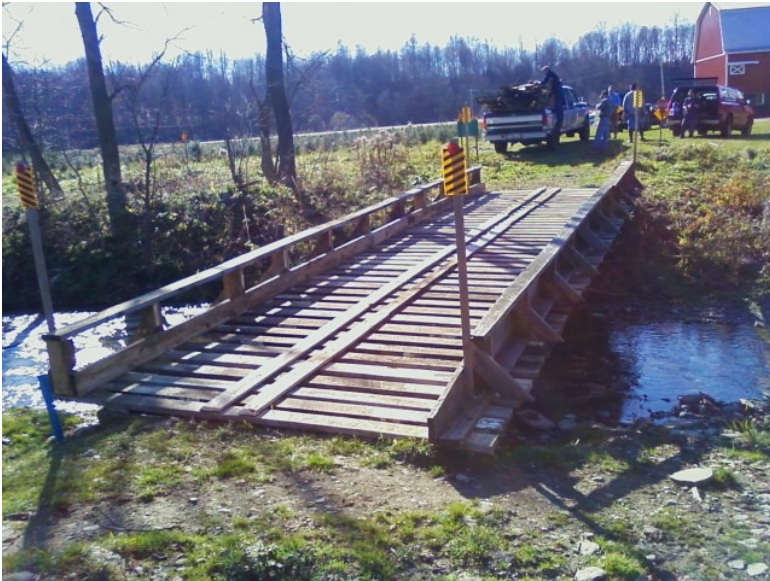
Bridge completely re-built on trail #1, at the Christmas Tree Farm, in Kennedy, corner of Rte 62 and 394
